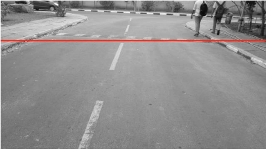
Fig.10: Example of undetected speed bump
